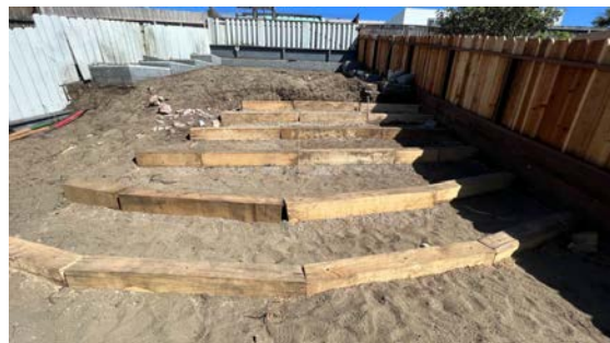
The SAS jobs are in their beginning stages and these stairs were installed recently. Portions will be cut out and a water feature will run through them.
